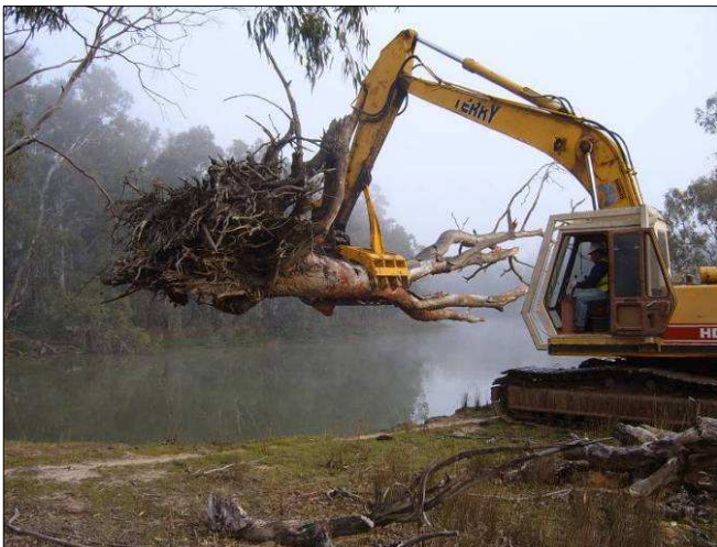
Resnagging works being conducted in the Murray River (Photo Credit: Martin Casey)
