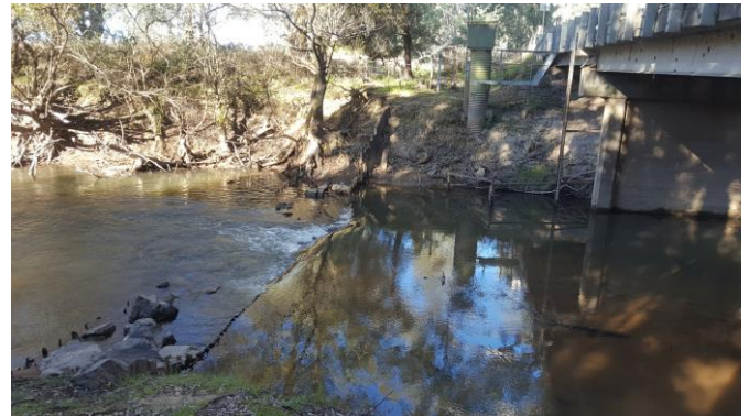
Figure 2: An ageing control structure requiring upgrade works (Photo: ARI)
