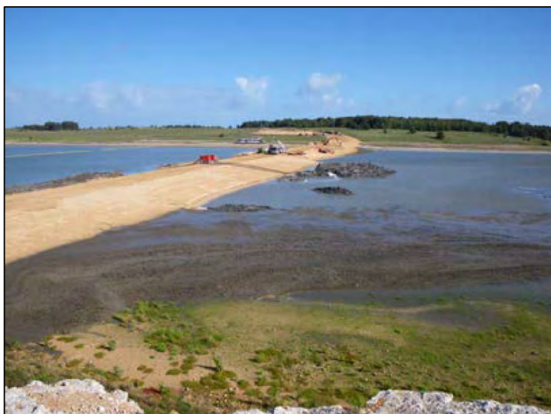
Figure 11. Earthen levee constructed across the Goolwa Channel separating the 'Goolwa weir pool' from the rest of Lake Alexandrina (photo: Chris Bice, SARDI)
