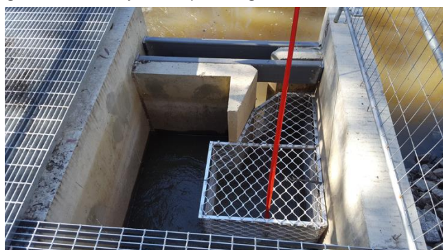
Figure 1 – The Chute fishway with aluminium fish trap installed (Photo: ARI)
